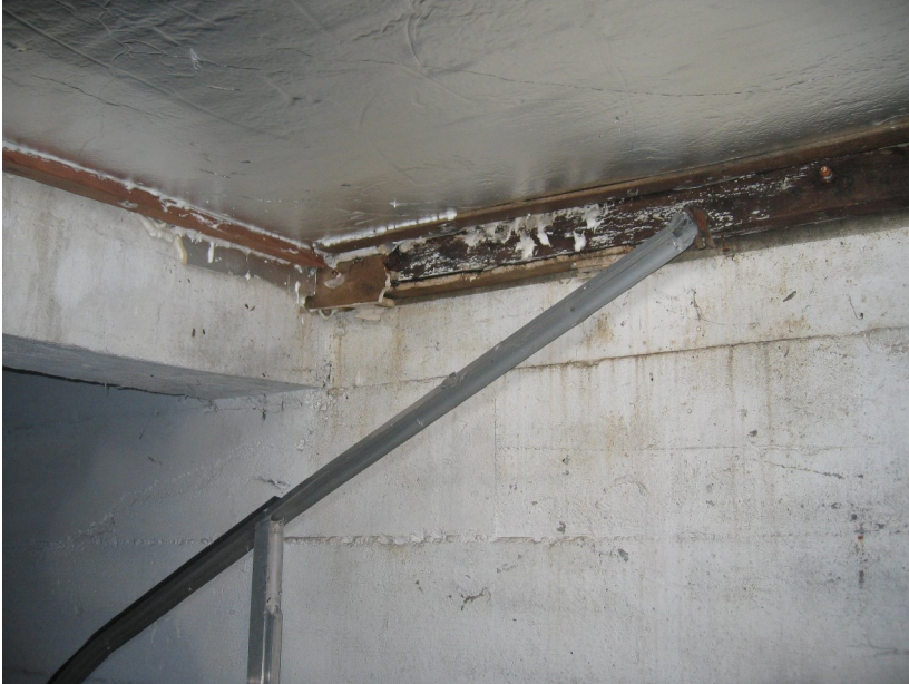
Garage wall with water saturated wood framing member at ceiling.
