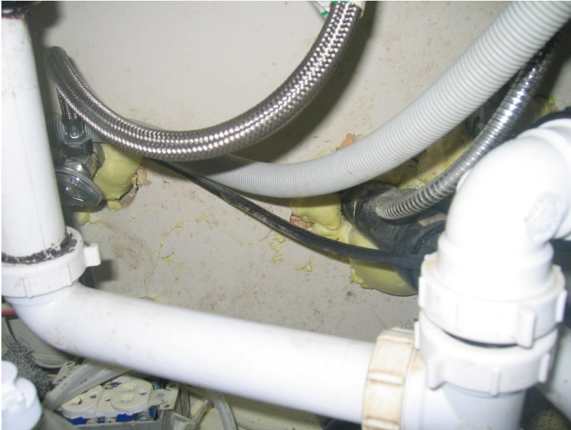
Under main kitchen sink back wall is damp with very small mold growth:
