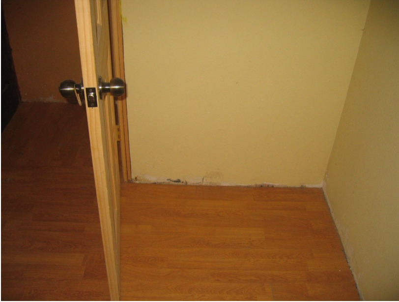
Downstairs hallway mold along bottom of wall:
