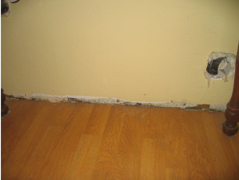
Downstairs laundry room mold along bottom of wall:
