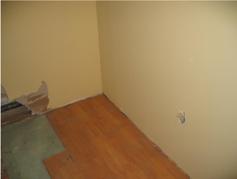
Downstairs spare room with mold along bottom of wall adjacent to laundry room:
