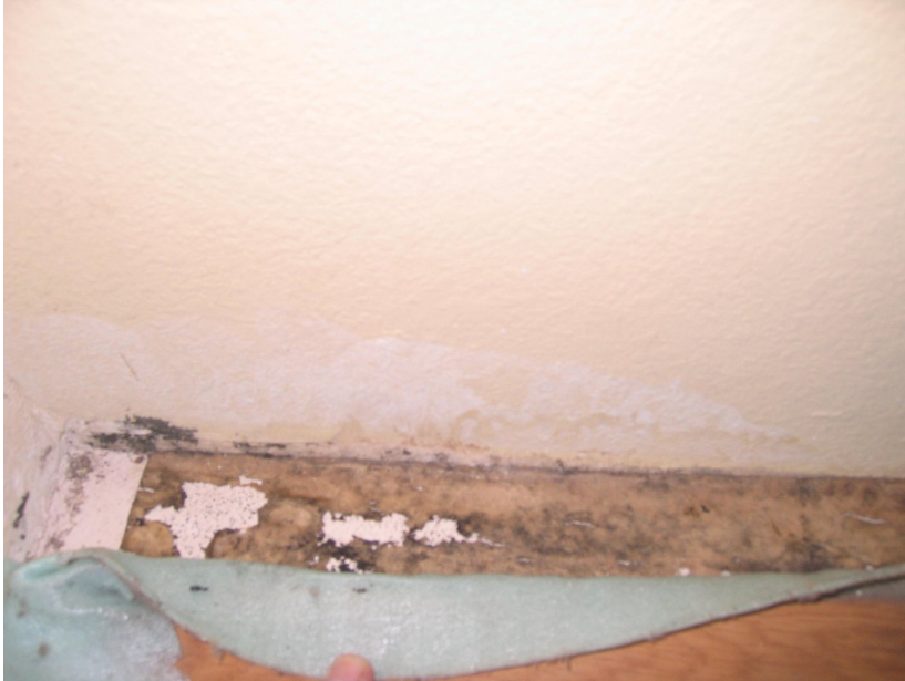
Downstairs laundry room mold under flooring and along bottom of wall:
