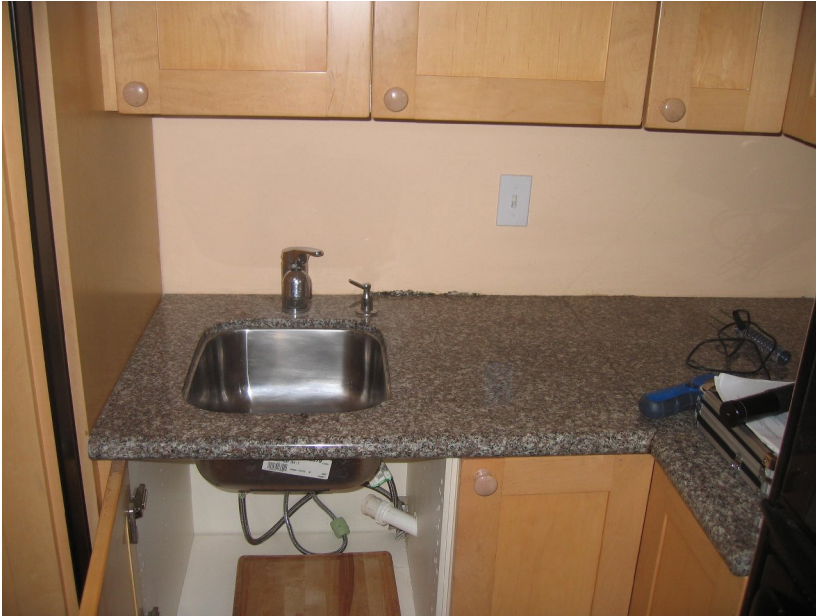
Secondary kitchen sink with mold on wall just above counter:
